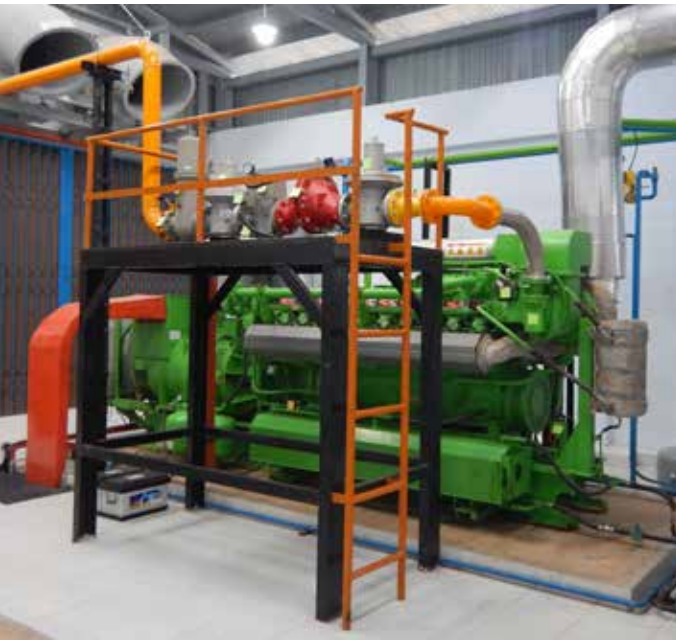
Biogas engine in Mukomuko
