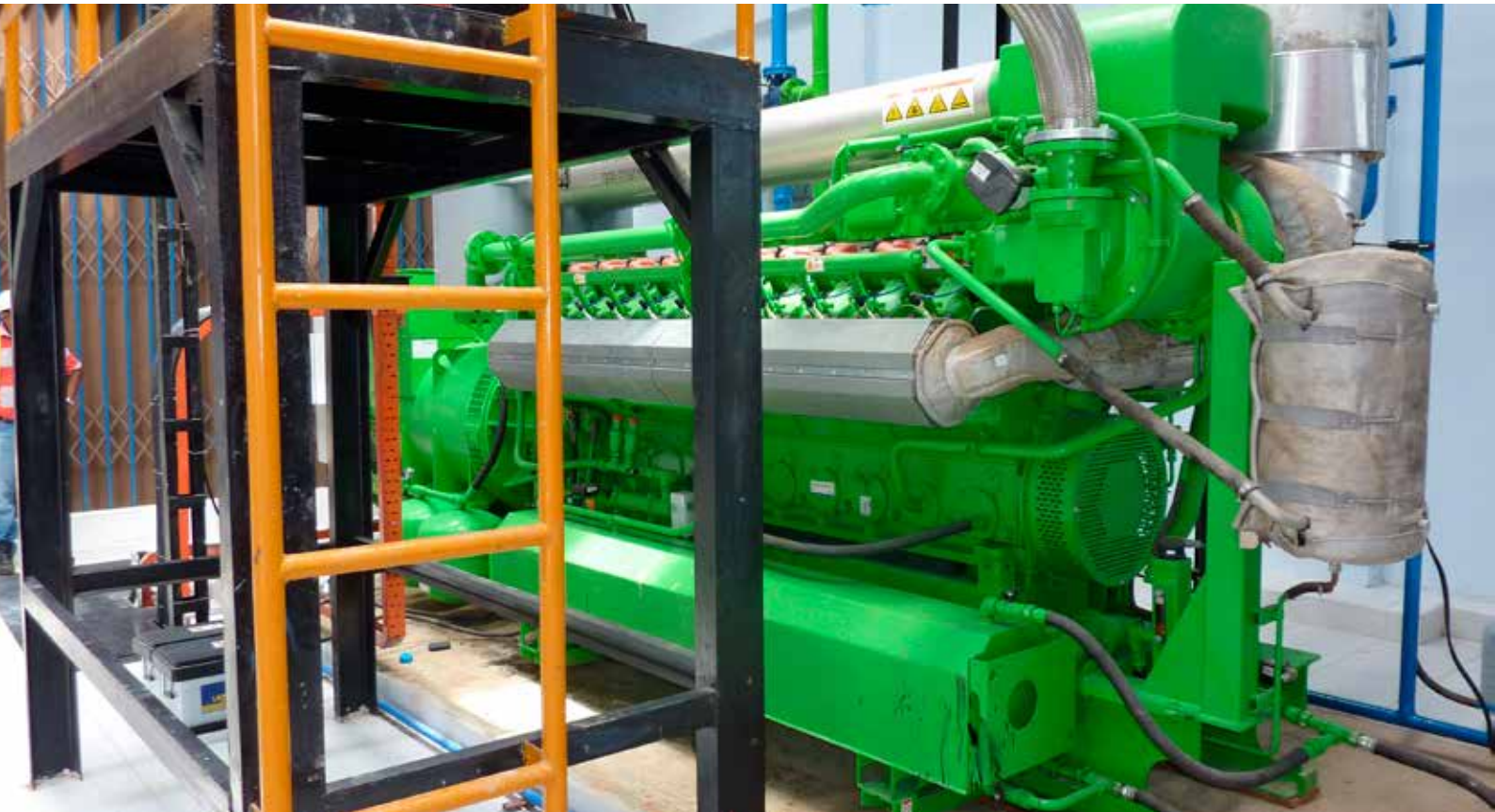
Biogas engine in Mukomuko Palm Oil Mill in Agro Muko in Bengkulu, Indonesia
