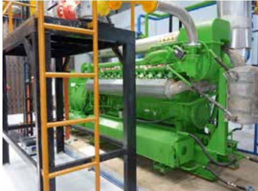
/// Close-up of a gas engine ///
