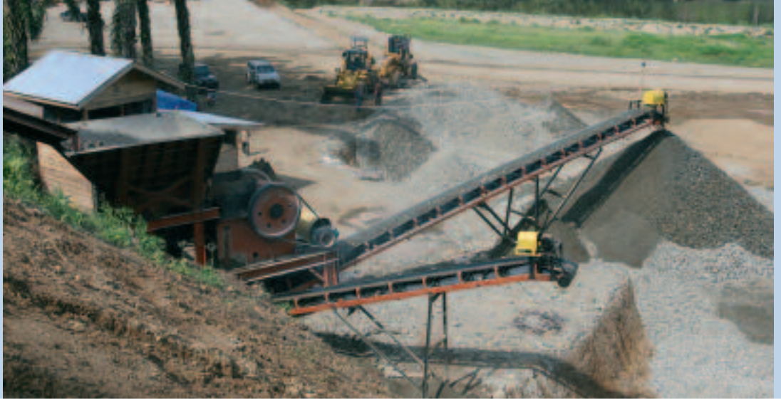
Stone crusher at Agro Muko
