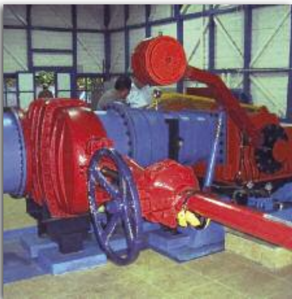
Hydraulic power station at Cibuni
