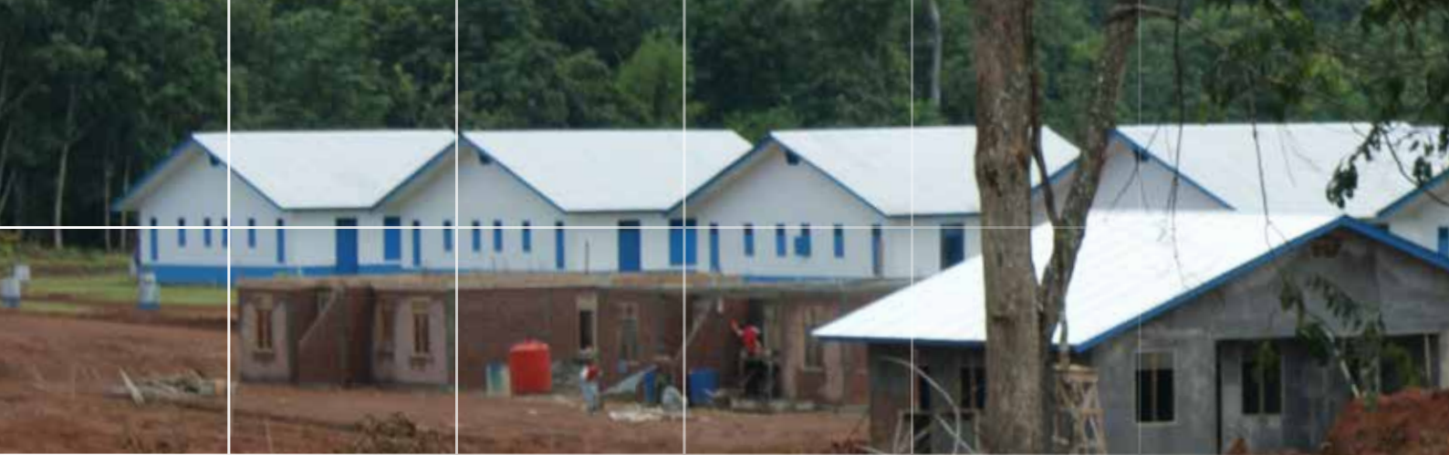
The construction of new workers' housing in Musi Rawas in South Sumatra
