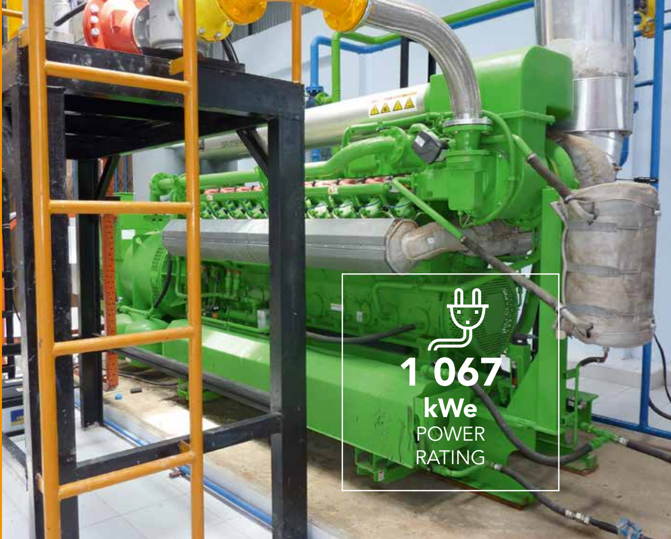
Close-up of the gas engine
